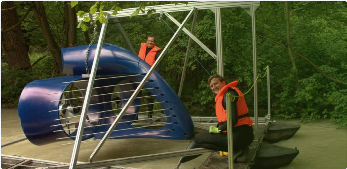
The Energyminer founders, Dr. Richard Eckl and Dr. Georg Walder, installing the Energyfish pre-series plant in Munich. Copyright: Energyminer GmbH
